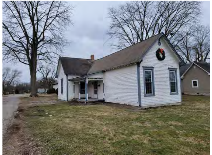
House at the corner of Southeastern Avenue and Clark Drive (Under Complete Renovation)
