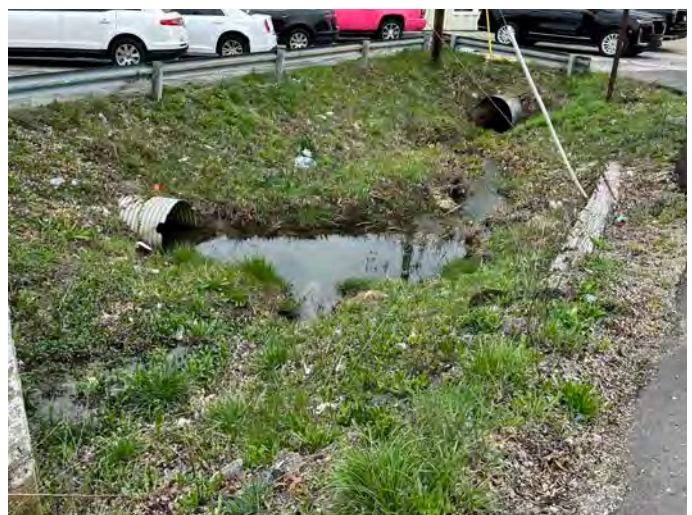
Open stormwater management ditch
