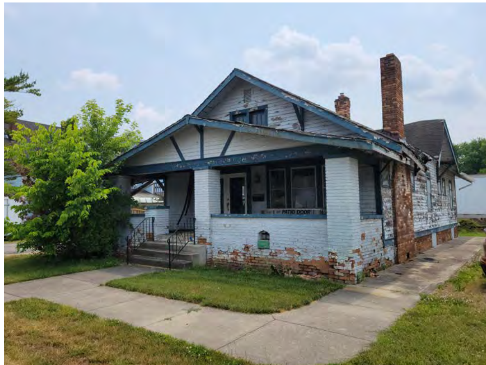
Dilapidated house on Southeastern Avenue, to soon be demolished.
