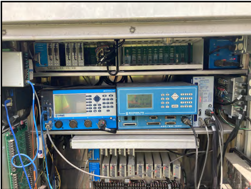
Looking Inside the Controller Cabinet Located in the Southeast Quadrant
