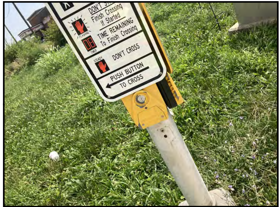
Pedestrian Button in Southeast Quadrant is in Need of Repair
