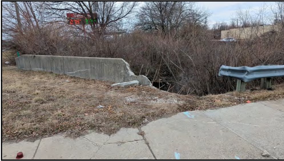
Damaged bridge headwall & guardrail in northwest quadrant
