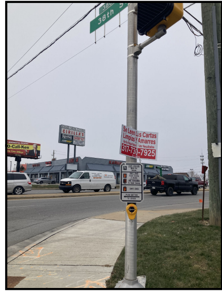
APS Pedestrian Signal - NE Quad (Installed mid 2022)
