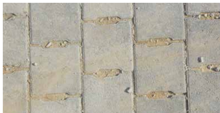
Clean permeable pavers (top) versus clogged (bottom)
