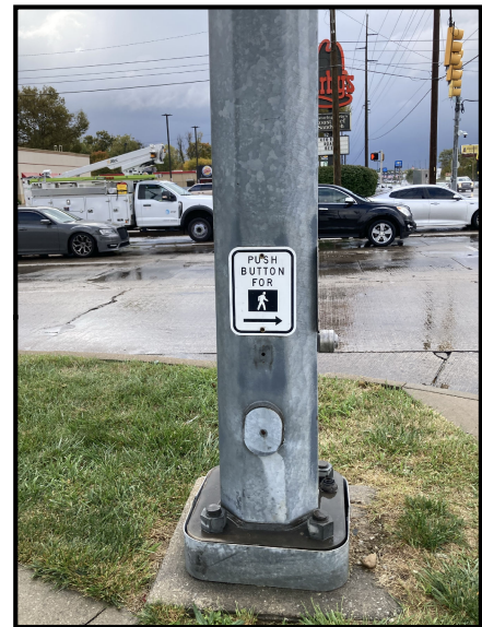
06 - Non-working pedestrian push button in NE quad
