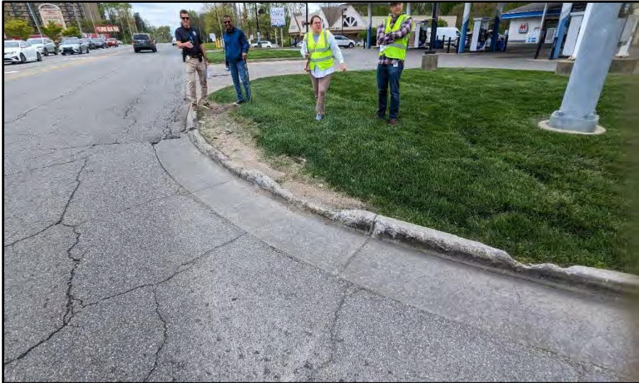
Photo 1 – Raised concrete curb in the northeast quadrant is being struck frequently due to alignment shift of Michigan Road.
