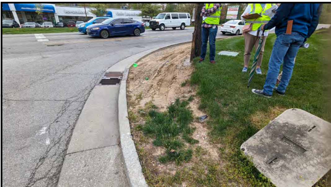
Over tracking of raised curb in the northwest quadrant.
