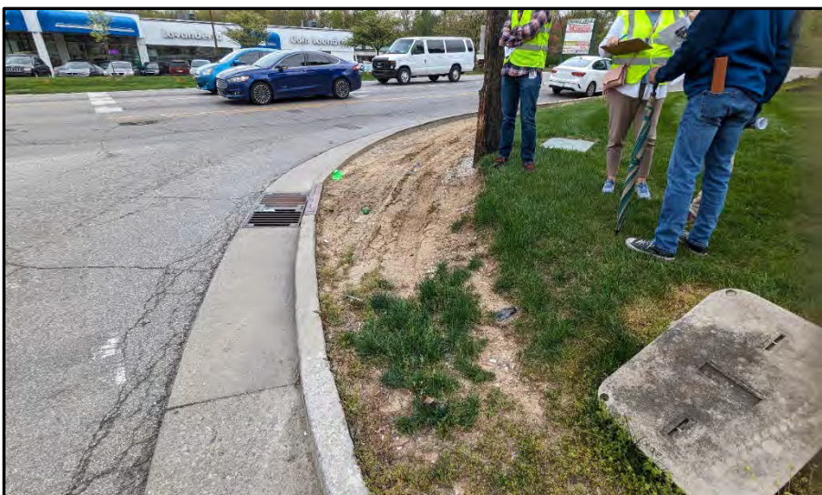
Photo 3 – Over tracking of raised curb in the northwest quadrant.
