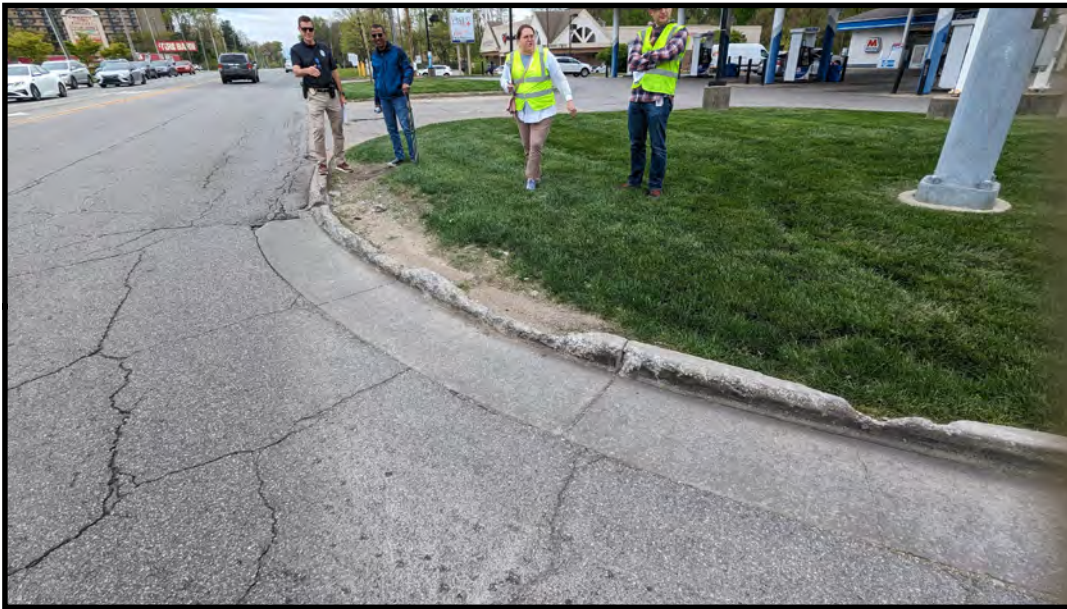
Raised concrete curb in the northeast quadrant is being struck frequently due to alignment shift of Michigan Road.
